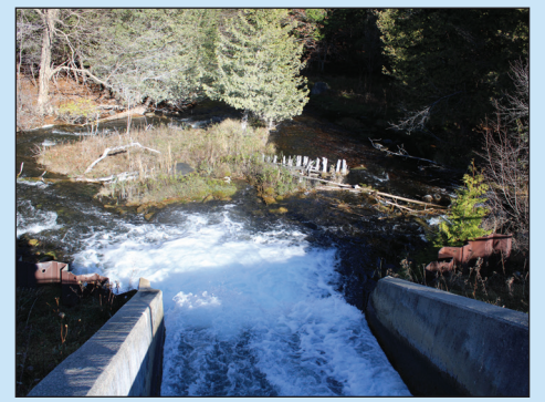
Rugg Pond concrete spillway feeding into Rapid River. Photos by Mark McAlpine
