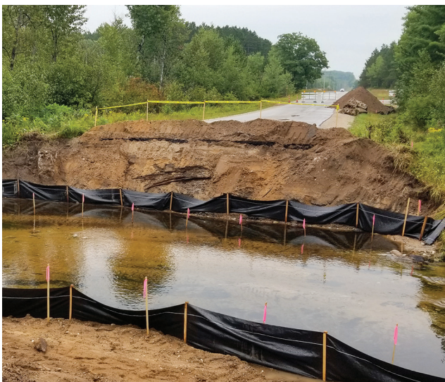
Construction begins on Robinson Road in late August with a Full-Channel timber Bridge coming soon.
