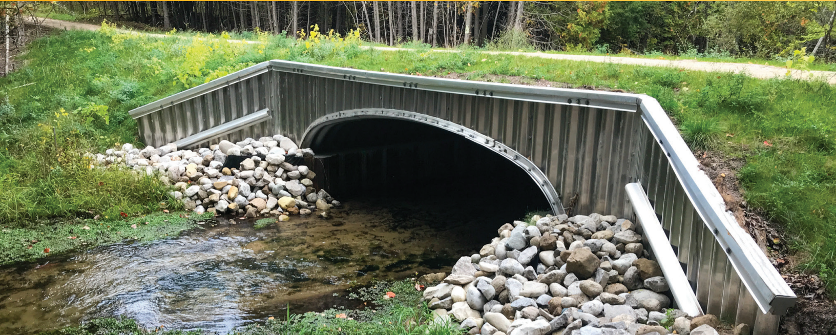
After: The Skinner Road crossing was upgraded to a wider, longer bottomless aluminum arch culvert, returning the natural width of the North Branch of the Platte as it flows under the roadway.
