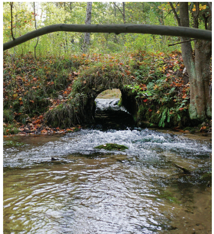
Before: An old, undersized boilerplate pipe was removed at the Skinner Road crossing over the North Branch of the Platte, clearing the way for a much larger culvert.
