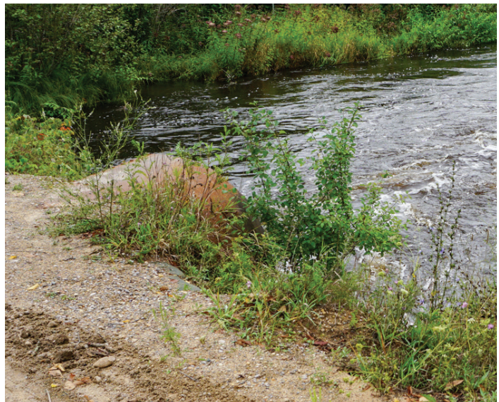
A narrow culvert in need of replacement on Fuller Road.
