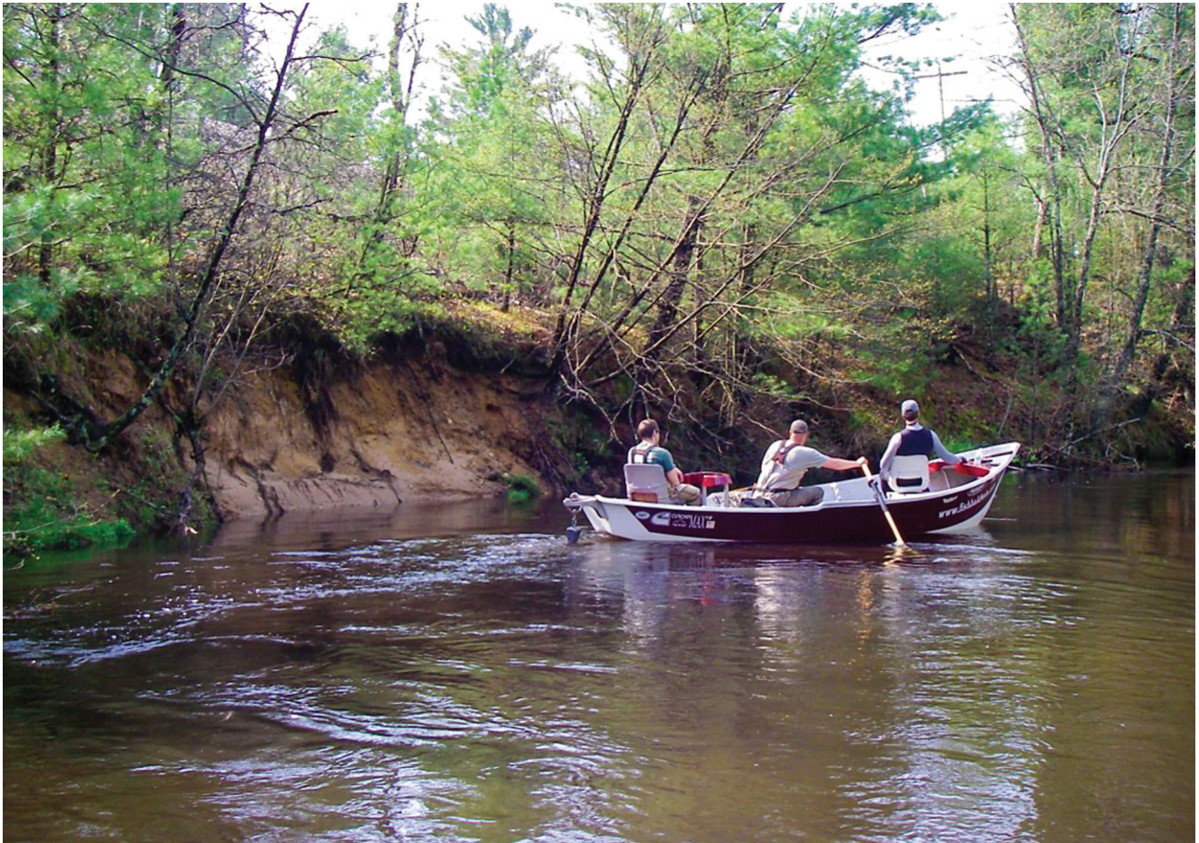
Anglers float by the eroding streambank at the Pere Marquette Railroad Stabilization Site.
