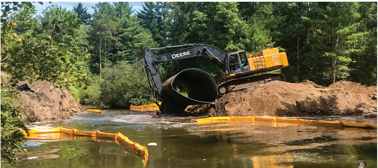
An excavator hauls away the old culvert from the Broomhead Road site back in early August. A new channel-spanning timber bridge will take its place.
